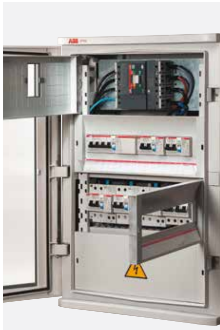
The blank and drilled panels are hinged onto both sides; the description of the installed components can be kept in the special compartment protected by a transparent, hinged flange.
